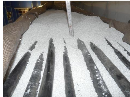
Picture B: Protected Cable Route
